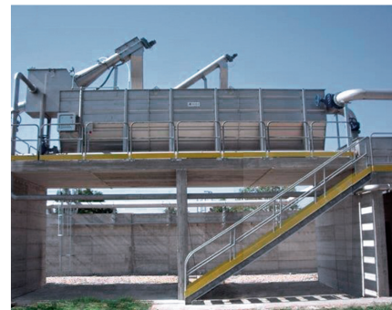
Municipal wastewater treatment plant
