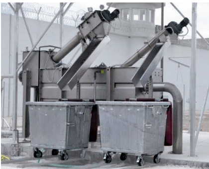
Prison wastewater treatment
